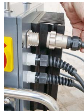
Figure 11b: Mains cable (unplugged)
